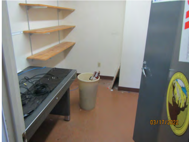
Photo 7 – Asbestos-containing brown resilient sheet flooring, 2 nd floor, northern offices
