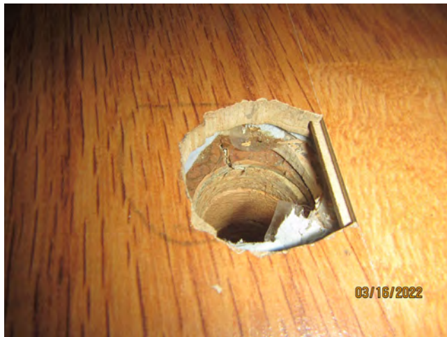
Photo 9 – Tan pebble-pattern resilient sheet flooring (beneath wood floor), 1 st floor, common area, southern offices
