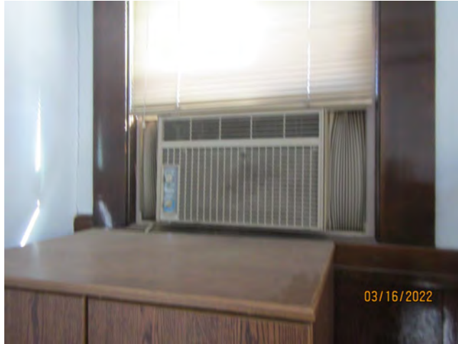
Photo 34 – Wall-mounted air conditioner, southeastern room, southern offices
