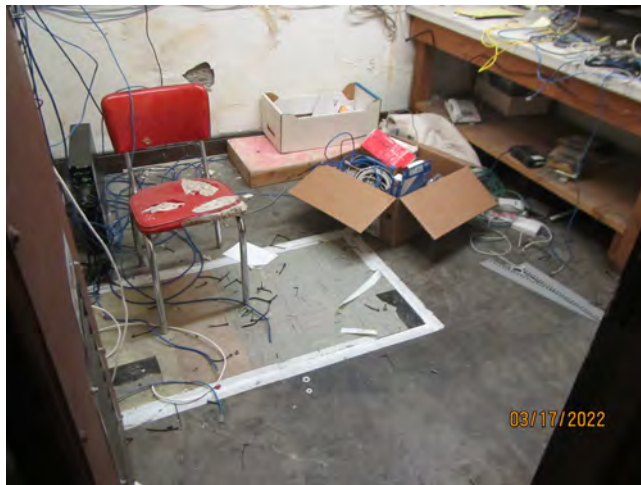
Photo 15 – Asbestos-containing multi-colored 9”x9” resilient floor tiles with black mastic, former IT room, basement, southern offices
