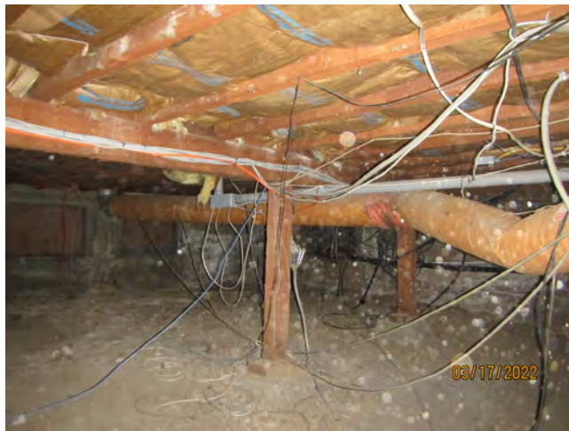
Photo 26 – Orange mineral wool duct, crawlspace, southern offices
