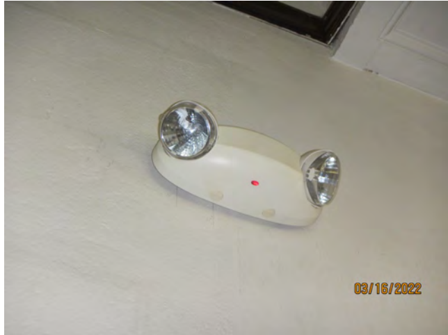
Photo 31 – Typical emergency light fixture with rechargeable batteries
