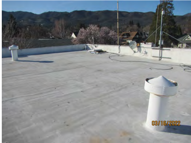
Photo 16 – Typical roof main field with underlying asbestos-containing silver paint and roof penetration mastic, southern offices
