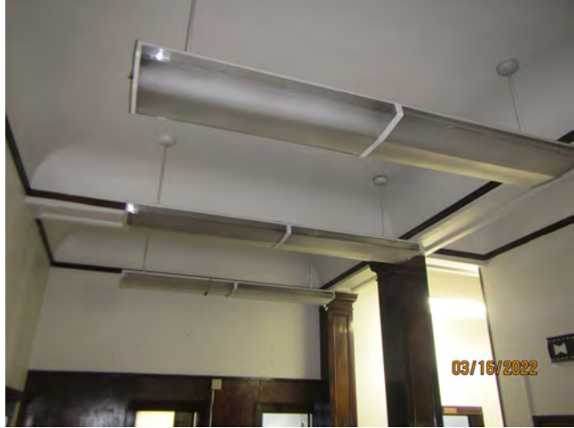
Photo 30 – Typical fluorescent light fixtures
