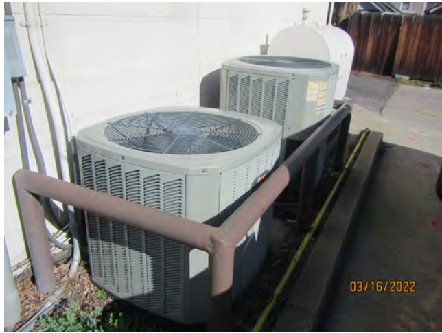
Photo 32 – Pad-mounted air conditioners, eastern exterior
