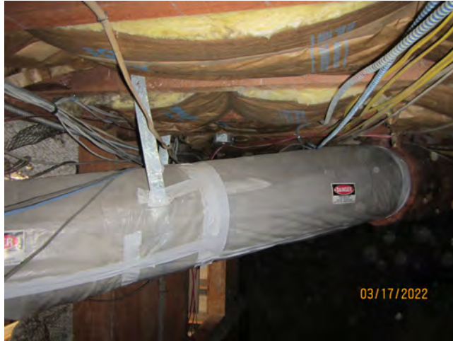
Photo 25 – Asbestos-containing paper duct wrap, crawlspace, southern offices
