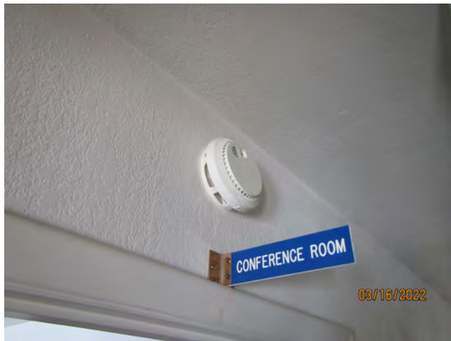
Photo 38 – Smoke detector, northern offices
