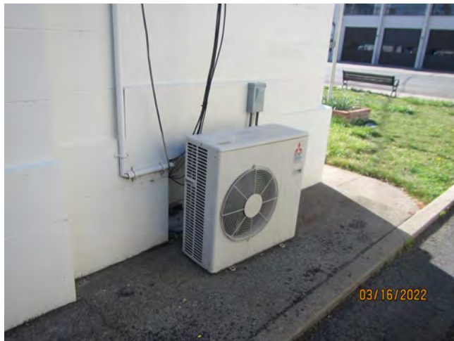
Photo 33 – Pad-mounted air conditioner, western exterior
