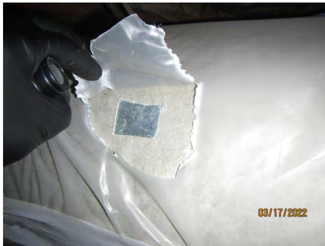
Photo 24 – Asbestos-containing paper duct wrap, crawlspace, southern offices
