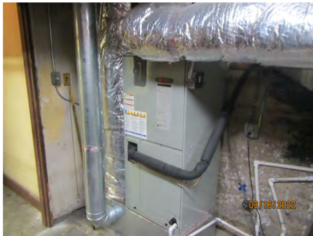
Photo 36 – HVAC units, basement, southern offices
