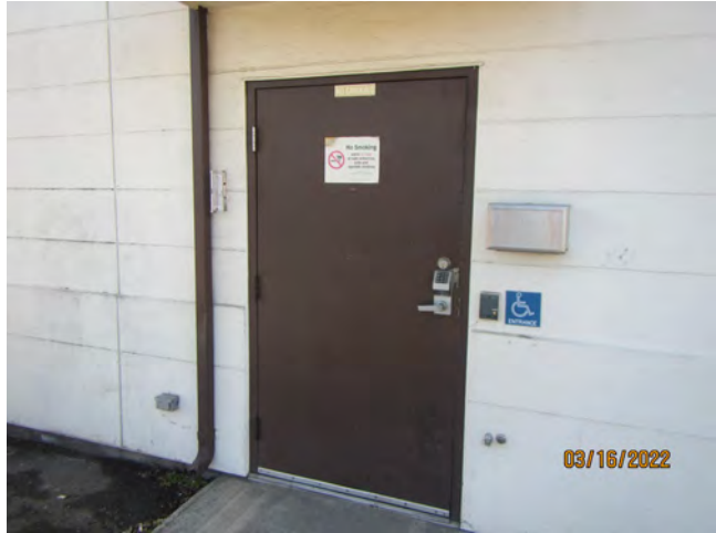
Photo 28 – Assumed asbestos-containing fire door, northern entrance, northern offices
