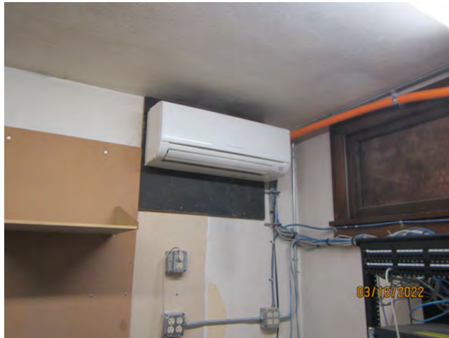
Photo 35 – Wall-mounted air conditioner, former IT room, basement, southern offices
