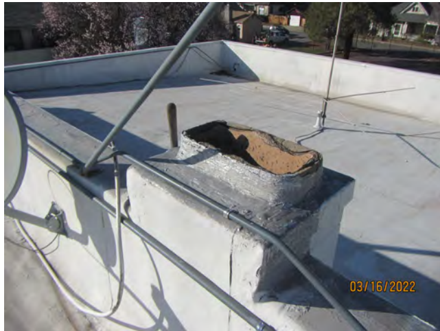
Photo 18 – Typical roof main field with underlying asbestos-containing silver paint and roof penetration mastic, northern offices
