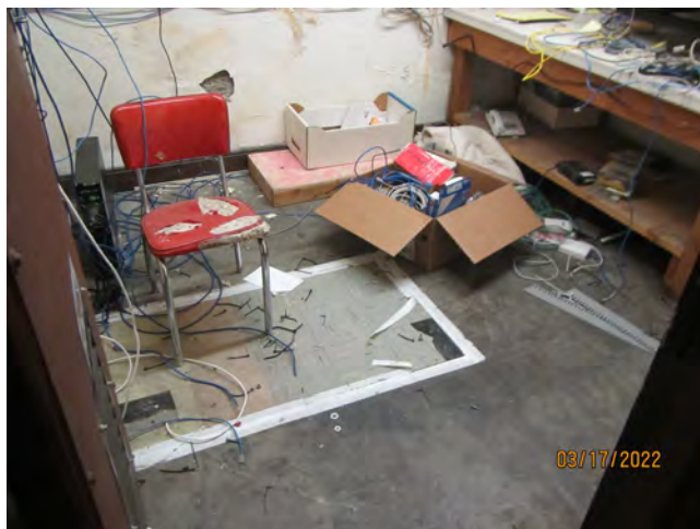
Photo 15 – Asbestos-containing multi-colored 9”x9” resilient floor tiles with black mastic, former IT room, basement, southern offices
