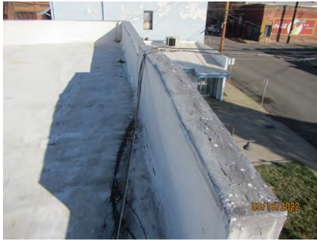
Photo 17 – Roof parapet with asbestos-containing mastic (cap) and underlying silver paint, southern offices
