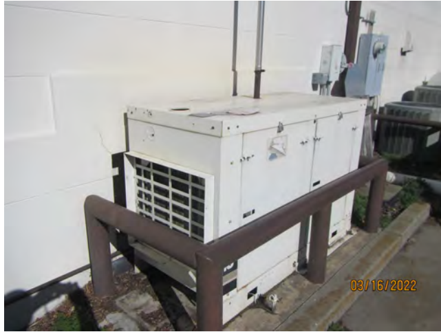
Photo 40 – Natural gas-powered auxiliary generator, eastern exterior
