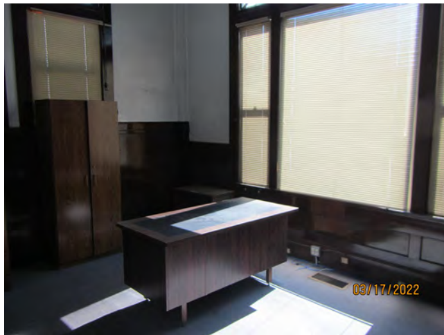
Photo 11 – Asbestos-containing gray carpet mastic, 1 st floor, southeastern and southwestern rooms, northern offices
