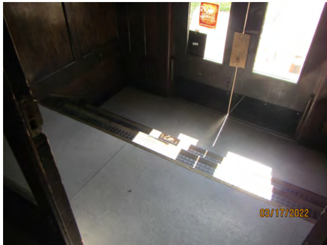
Photo 12 – Gray resilient sheet flooring and brown stair tread, 1 st floor entrance, southern offices
