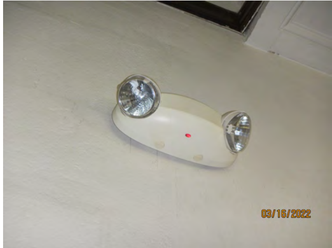
Photo 31 – Typical emergency light fixture with rechargeable batteries
