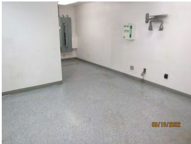
Photo 5 – Gray 12''x12'' resilient floor tile with brown mastic, 1 st floor, northern offices
