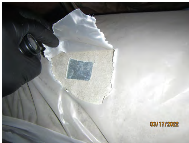
Photo 24 – Asbestos-containing paper duct wrap, crawlspace, southern offices
