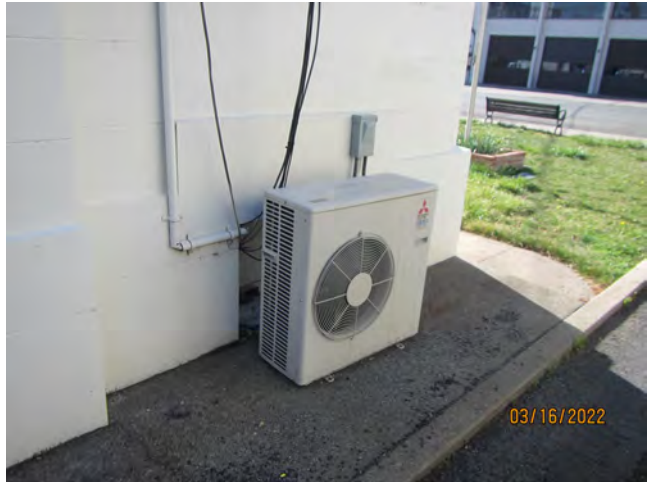
Photo 33 – Pad-mounted air conditioner, western exterior
