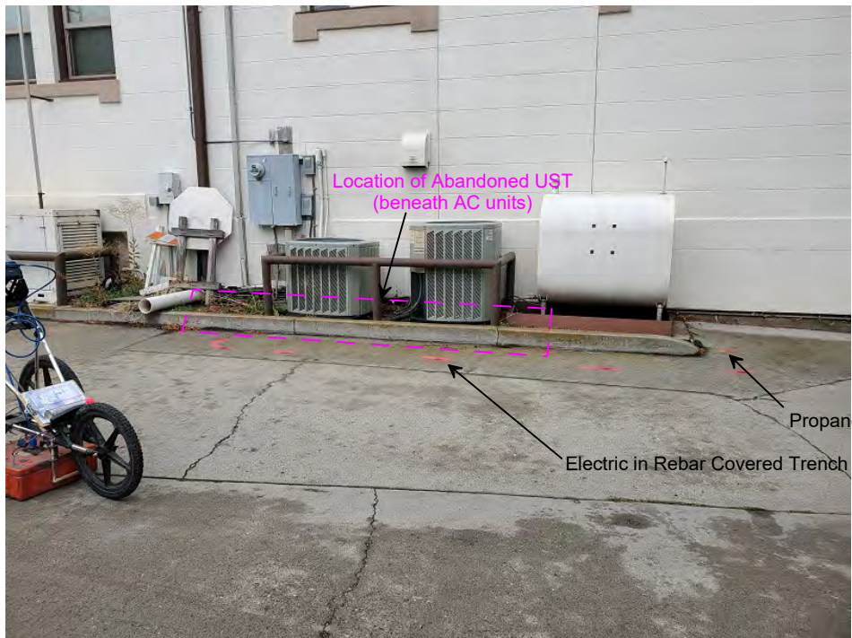
Photograph Showing Location of Abandoned UST Beneath AC Units
