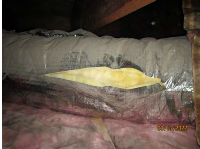
Photo 29 – Yellow fiberglass flex-duct and pink fiberglass batting insulation, ceiling cavity, northern offices
