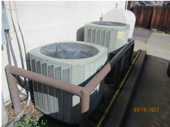
Photo 32 – Pad-mounted air conditioners, eastern exterior
