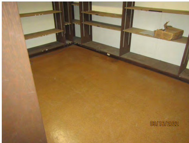
Photo 6 – Asbestos-containing brown resilient sheet flooring, 1 st floor, northern offices, northwestern office
