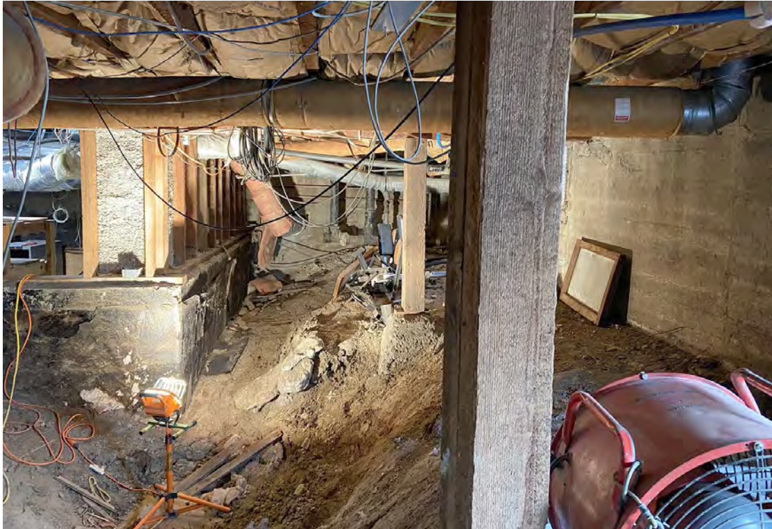
Photo No. 3 Utility conduits and trenching/excavation area in unfinished portion of basement
