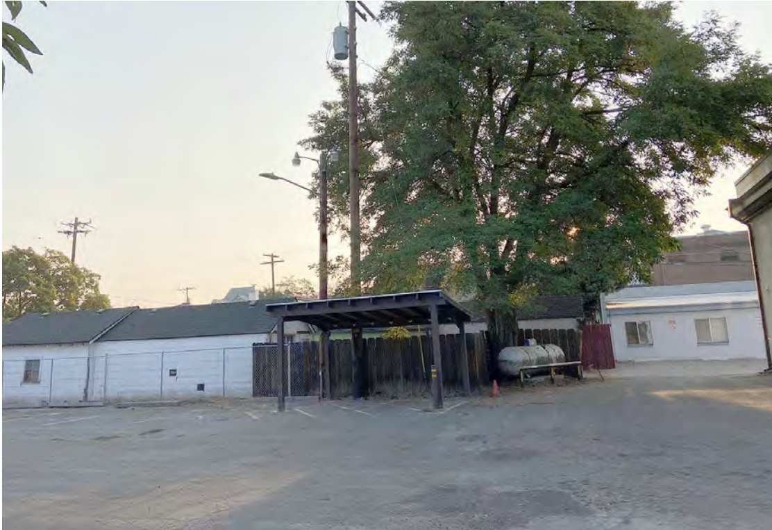
Photo No. 9 View to the east of propane AST and pole-mounted transformer in central portion of the Site
