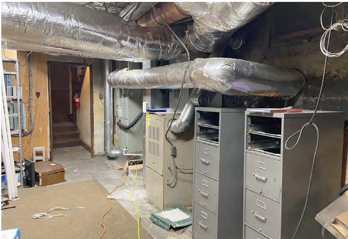
Photo No. 4 Furnace and air conditioning in the finished portion of the basement
