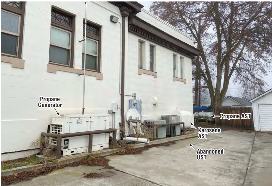
Photo No. 8 Propane powered generator and concrete patching over UST on the east side of the site building
